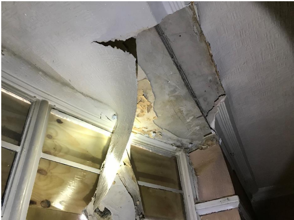
Roof leak / collapsing ceilings
